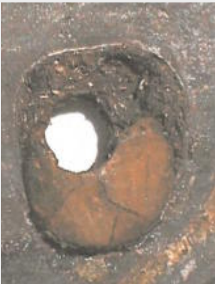
Close-up view of a failed water feed- through opening
